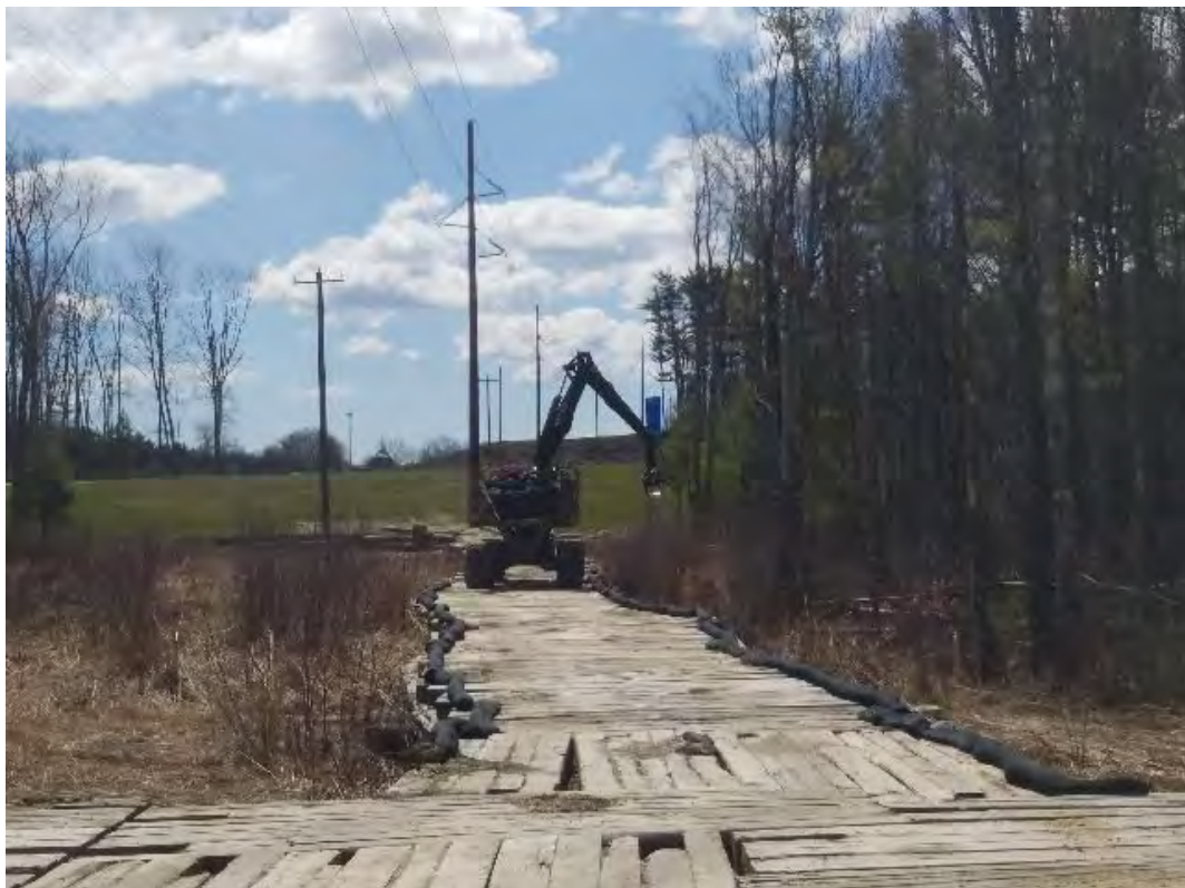
Fig 6: Removing timber mats used for access road to Strs. 117-118 in wetland NW9. Viewing southeast. (04-17-20).
