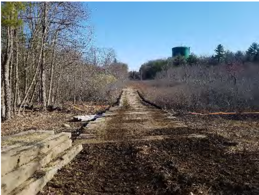
Fig 4: Installing timber mats for access road to Str. 35, through wetland DW41. Viewing north. (04-17-20).
