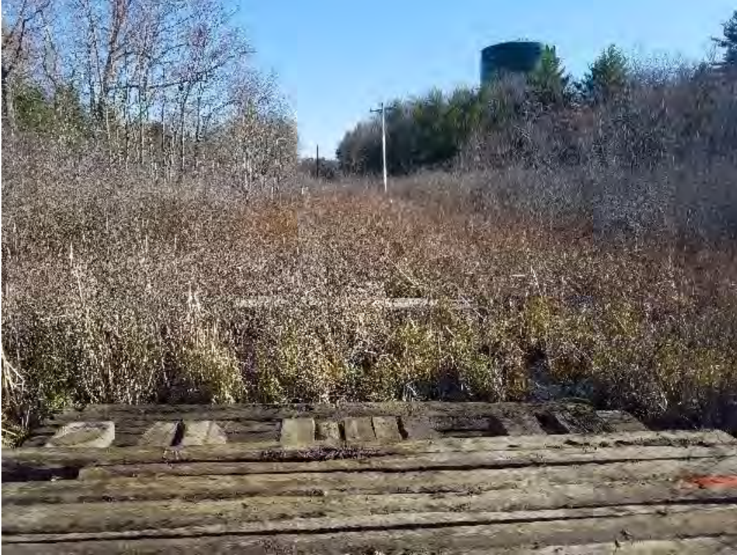
Fig 5: Installing timber mats for access to Str. 35, through wetland DW41. Viewing north. (04-17-20).
