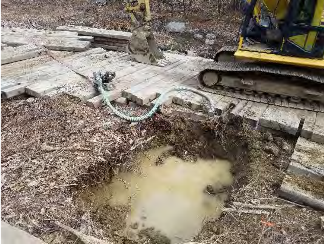
Fig 19: Setting up pump to dewater groundwater in Str. 89 foundation hole. Viewing north. (04-20-20).
