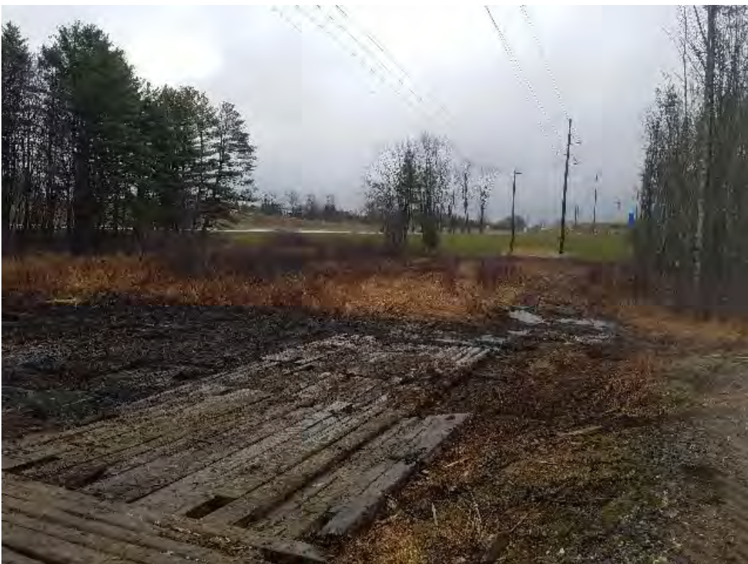
Fig 14: Continuing to remove timber mats around Strs 117-118 in wetland NW9. Viewing southeast. (04-18-20).
