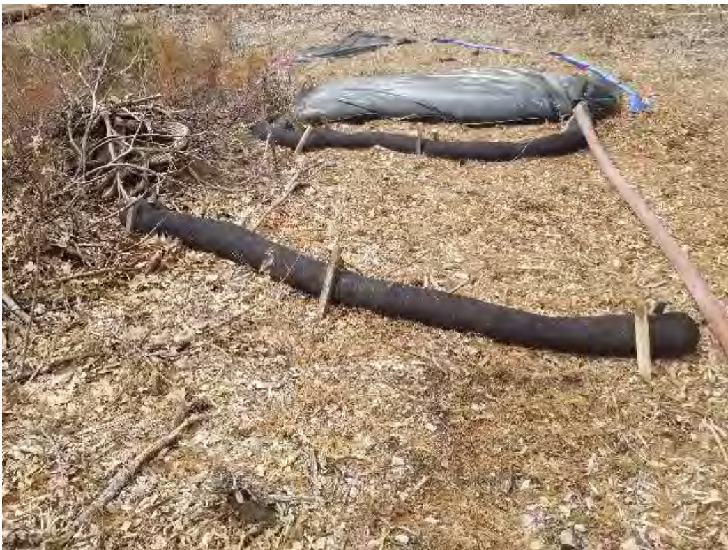
Fig 20: Filter bag and downslope BMPs installed for dewatering groundwater from Str. 89 foundation hole. Viewing northwest. (04-20-20).
