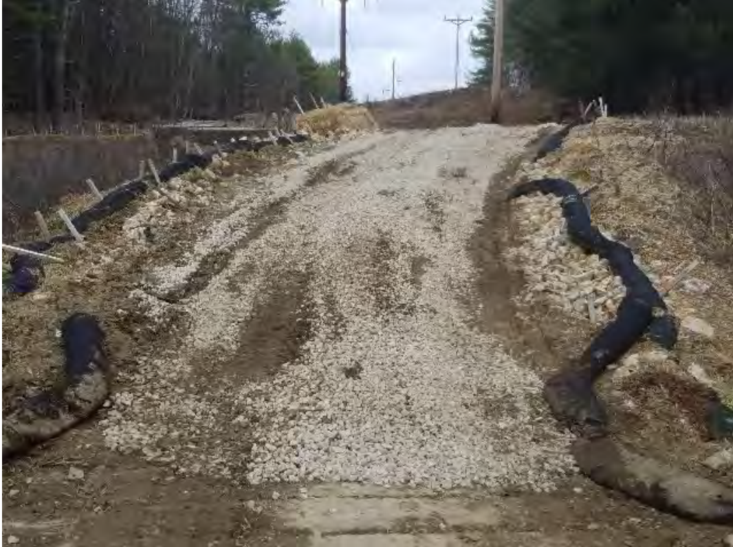
Fig 29: Stone installed on eastern slope of access road between Strs. 51 and 52. Viewing northeast. (04-22-20).
