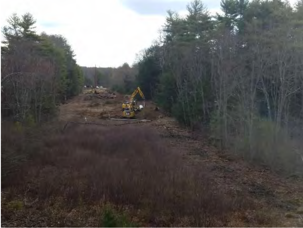
Fig 3: Excavating foundation for Str. 82. BMPs installed between work site and wetland DW38. Viewing east. (04-16-20).
